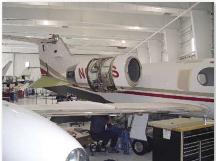
The two photos above were shot at West Star Aviation’s facility in Colorado during the installation of the Raisbeck ZR LITE Performance System and Aft Fuselage Locker on AirMed’s Lear 35.
